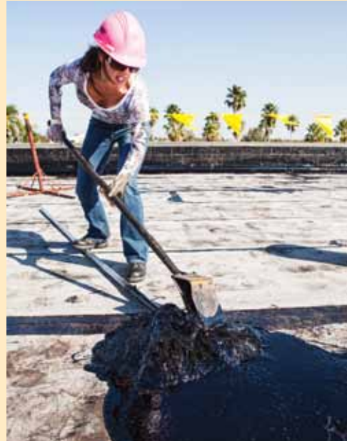
› Naomi Dupre of Kirby Fiberglass demonstrates how to scrape excess asphalt out of a mop. Photo: Redinger-Libolt.
