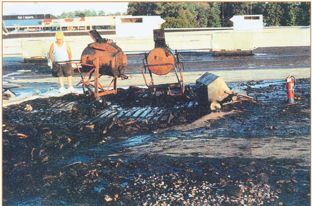
This fire at a large mall in the Southeast started as the result of spontaneous combustion of a roofing mop used earlier in the day.
