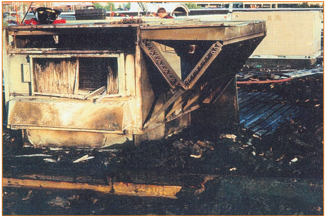
HVAC equipment on the roof of the mall destroyed by the fire.
